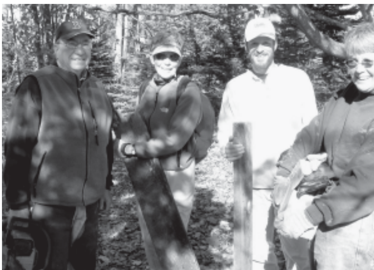
Bob Miller, Sue Owen, Michael Burgess, and Gail White repair bridges at Sklar Park.
